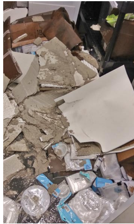
This not an art installation! This is the work of a tired hot water heater given a weekend to do its damage. It's the kind of work no one wants to see happen to them.
